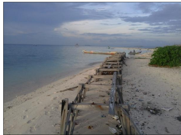
research in 2008. Fig. 5. Seawall made of wood damaged as a result waves hit in the west season
