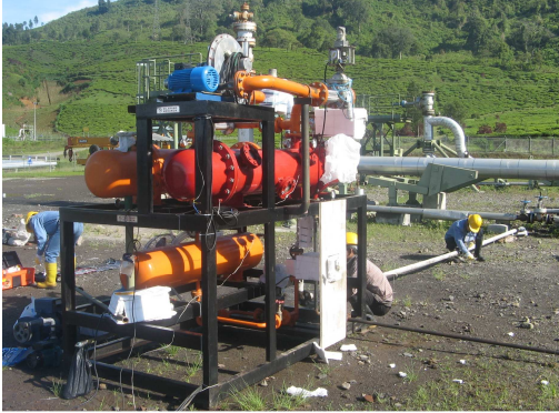
Figure 2. Installation of 2 kW binary cycle power plant model, Bambang Teguh P. et. al (2010)
