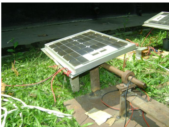
Fig. 5. Photographic of Experimental set-up of the Fixed Panel
